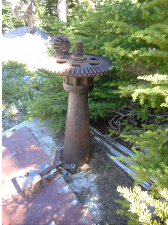
Photo 8 – Lower Klonaqu Lake Gate Actuator (Gate Chamber Access Lid Visible)
