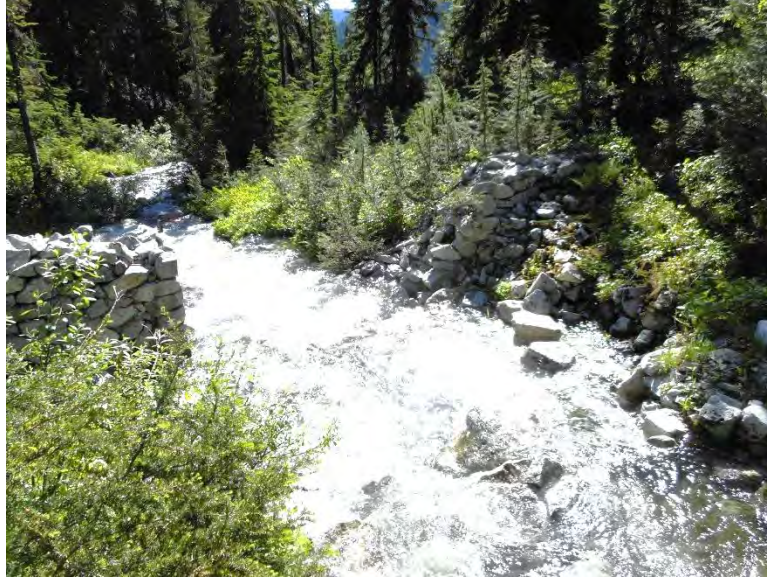
Photo 5 - Square Lake Flow with Gate Open (Destroyed Weir Visible)
