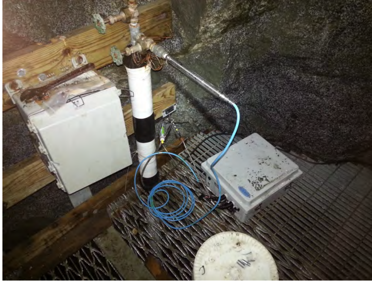
Photo 35 - Upper Snow Lake Outlet Works - Pressure Monitoring Equipment
