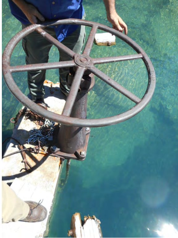
Photo 19- Colchuck Lake Gate Actuator
