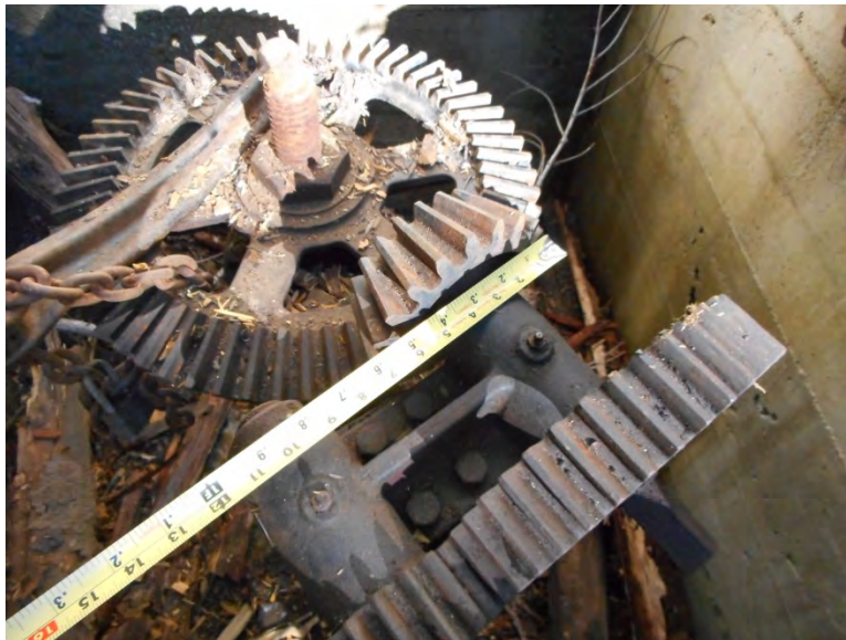
Photo 2 - Square Lake Gate Actuator
