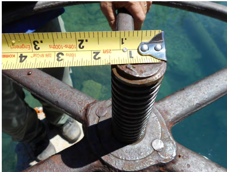
Photo 20 - Colchuck Lake Gate Actuator Stem (After Operation)
