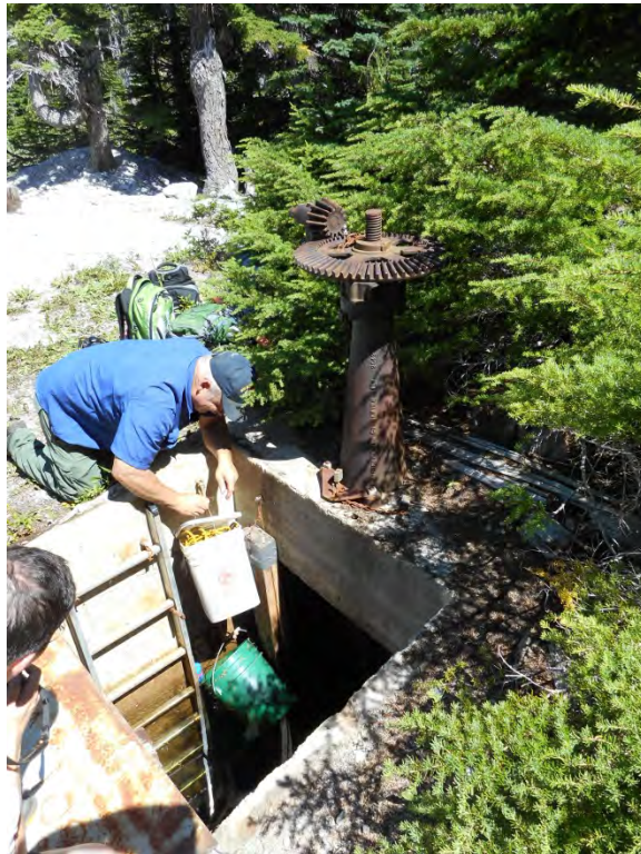
Photo 9 - Lower Klonaqu Lake Gate Chamber Open with Gate Actuator
