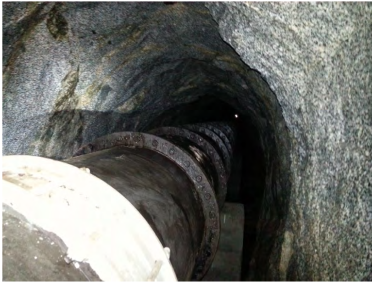
Photo 34 - Upper Snow Lake Outlet Works - 30" Diameter Pipe in Tunnel, View Looking Downstream
