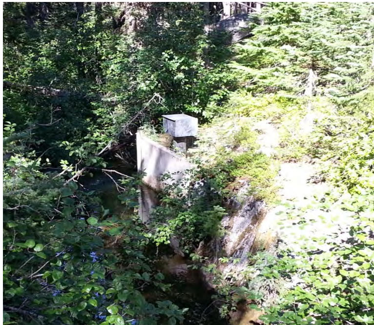
Photo 40 - Nada Lake Parshall Flume Stilling Well / Monitoring Equipment Housing (View of South Side from Upstream / North Side)
