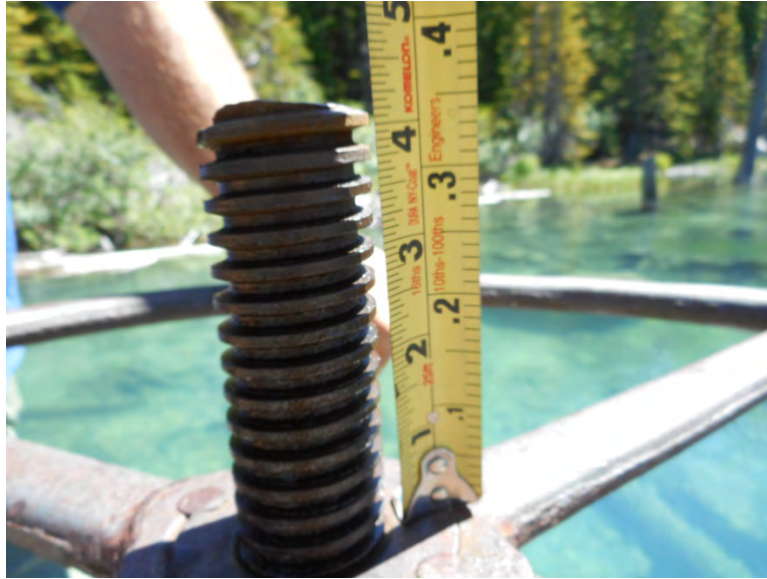
Photo 21 - Colchuck Lake Gate Actuator (After Operation)
