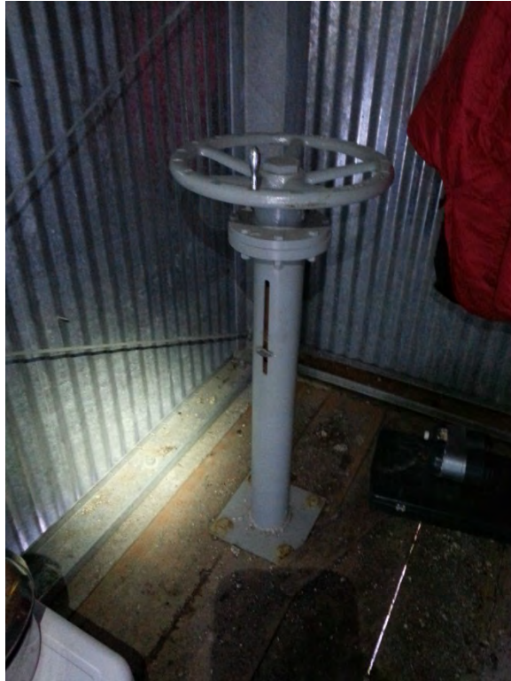
Photo 29 - Upper Snow Lake Outlet Works - Butterfly Valve Actuator
