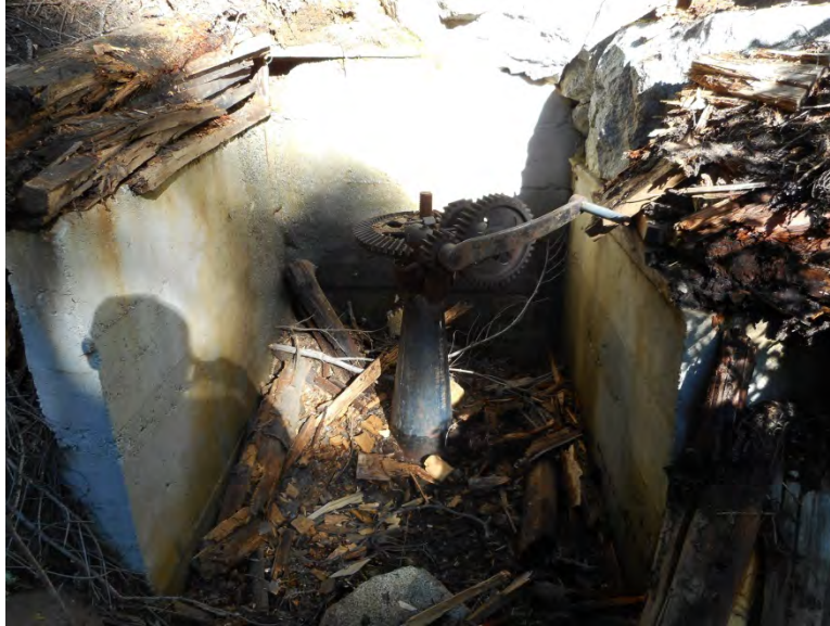
Photo 1 - Square Lake Gate Actuator
